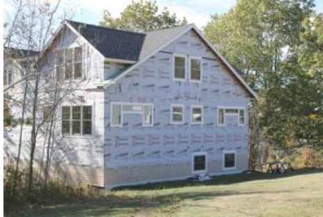
The back and side view of the three-unit building, which should be finished in January.
